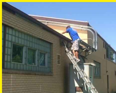
Brian Yost of All About Guttering, replaced 50 year old guttering with 5" commercial guttering and downspouts on the exterior of the school.
