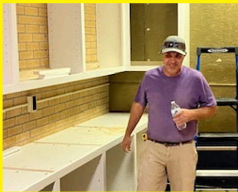
As part of the Capital Improvements, a new concession room has been created in place of a former storage room.
